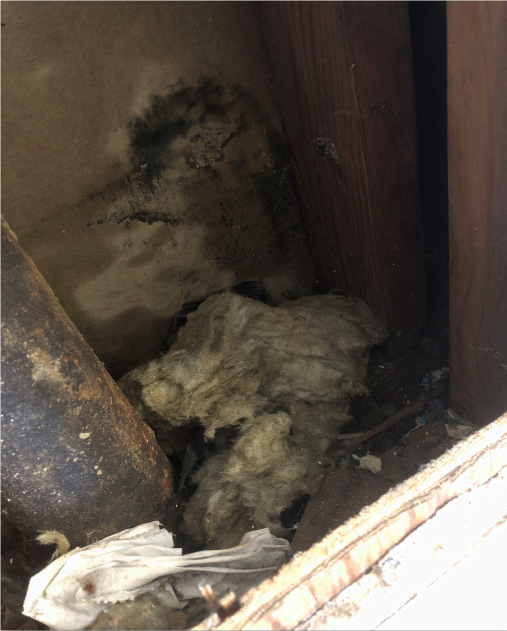
Black Mold Found in the Wall:
