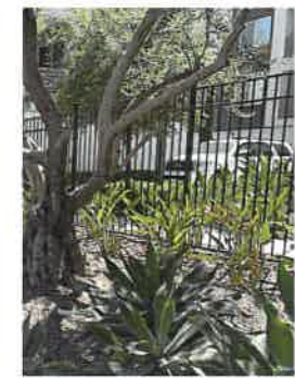
EXISTING TUBULAR STEEL FENCE
